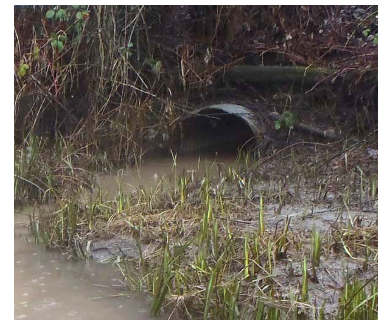
Outfall discharging turbid water into Johnson Lake
